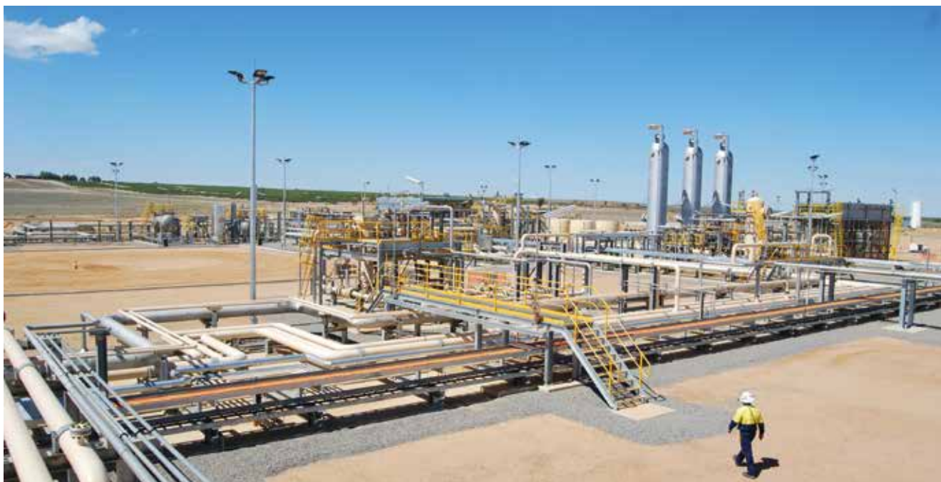
Storage capacity at APA's Mondarra Gas Storage Facility was increased during FY2016 with the completion of a new injection/withdrawal well.
